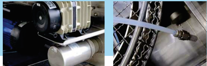
Oxygen membrane compressor
